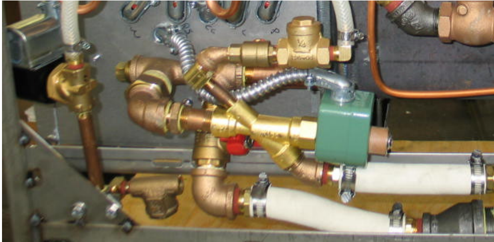
Figure 3 Layout for Drain for 24” Boiler Shown Installed
