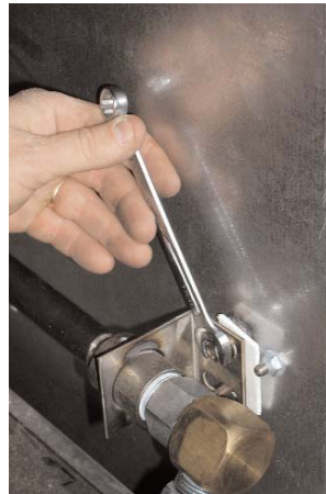
9. Remove gas line hold down bracket.
