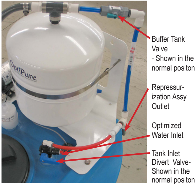
50 Gallon Storage Tank
