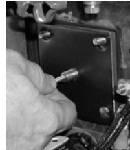
STEP 5 PULL CLAMP BAR STUD THROUGH BLOCK-OFF WHILE POSITIONING BLOCK-OFF PLATE OVER REMAINING STUDS.
