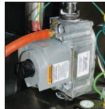
7. Gas Valve (showing hose for pressure tap)
